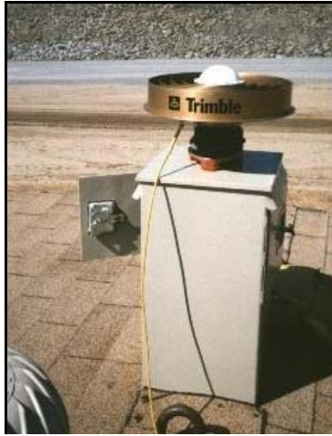
Figure 7. Choke ring antenna on observation shelter roof.
